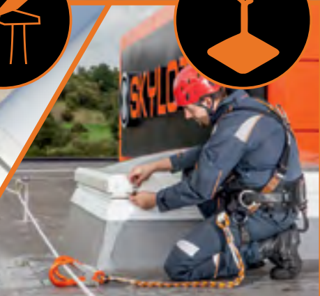
Permanent Fall Protection / Architecture
